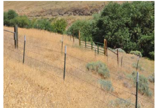
Fencing installed with funds from the Conservation Commission and Department of Ecology. Photo by Jodi Prout
